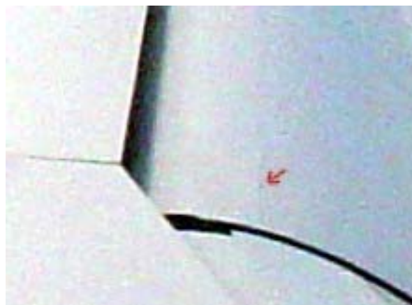
Photo 5. Possible point of origin of fracture
